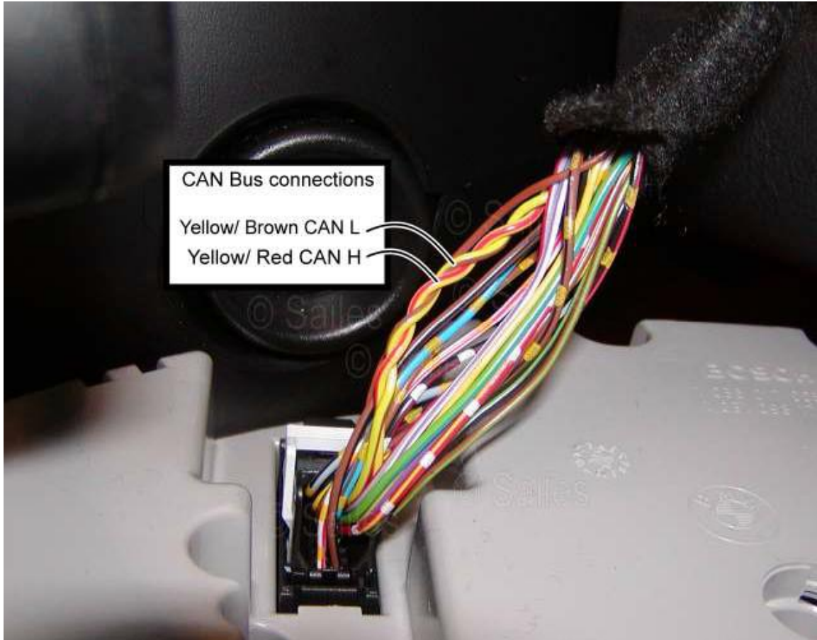
Picture from New Model BMW 3 series Wiring on rear of instrument cluster
